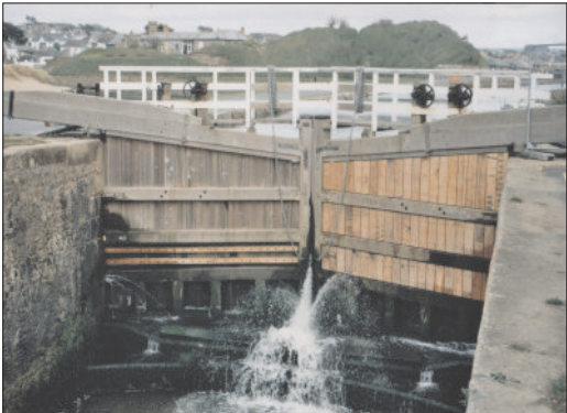
The Sea Lock with cladding on the right hand gate only. Photo Chris Jewell
