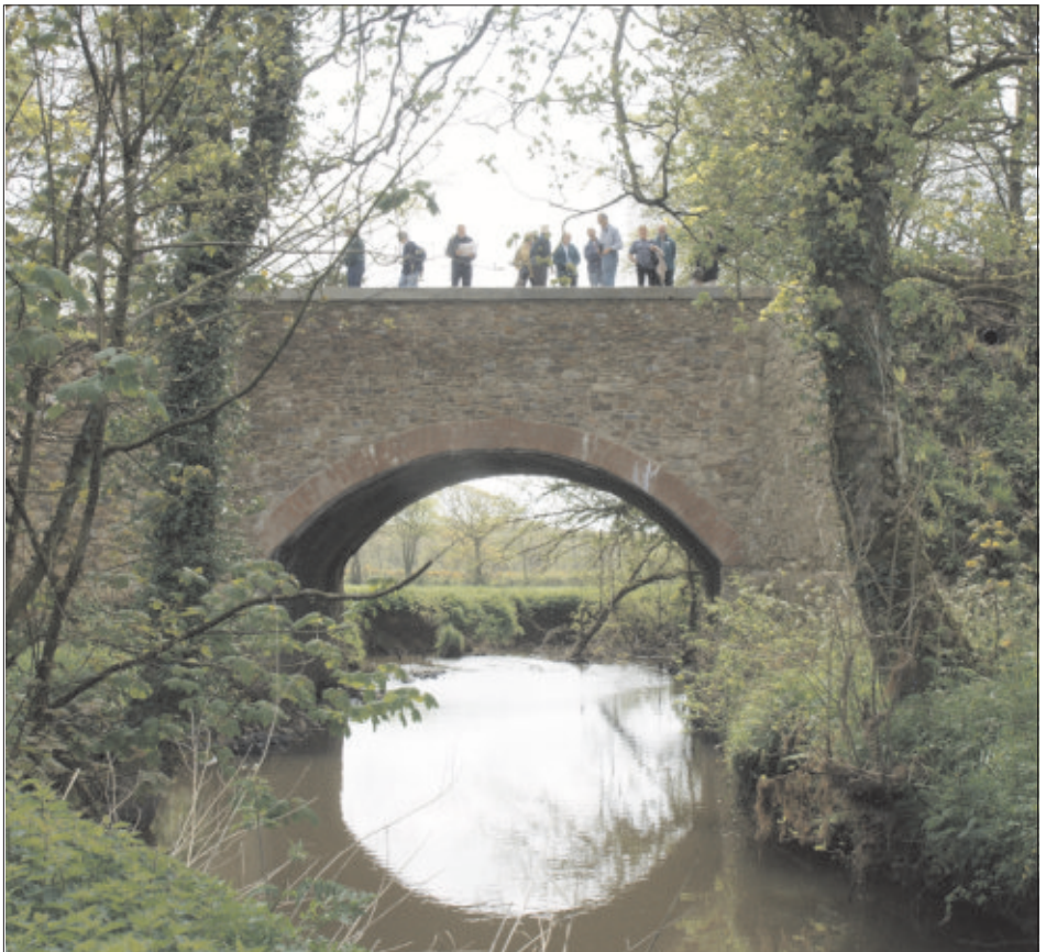
Visitors on the IWA South West Region AGM weekend inspecting Burmsdon Aqueduct. Photo Mike Moore
